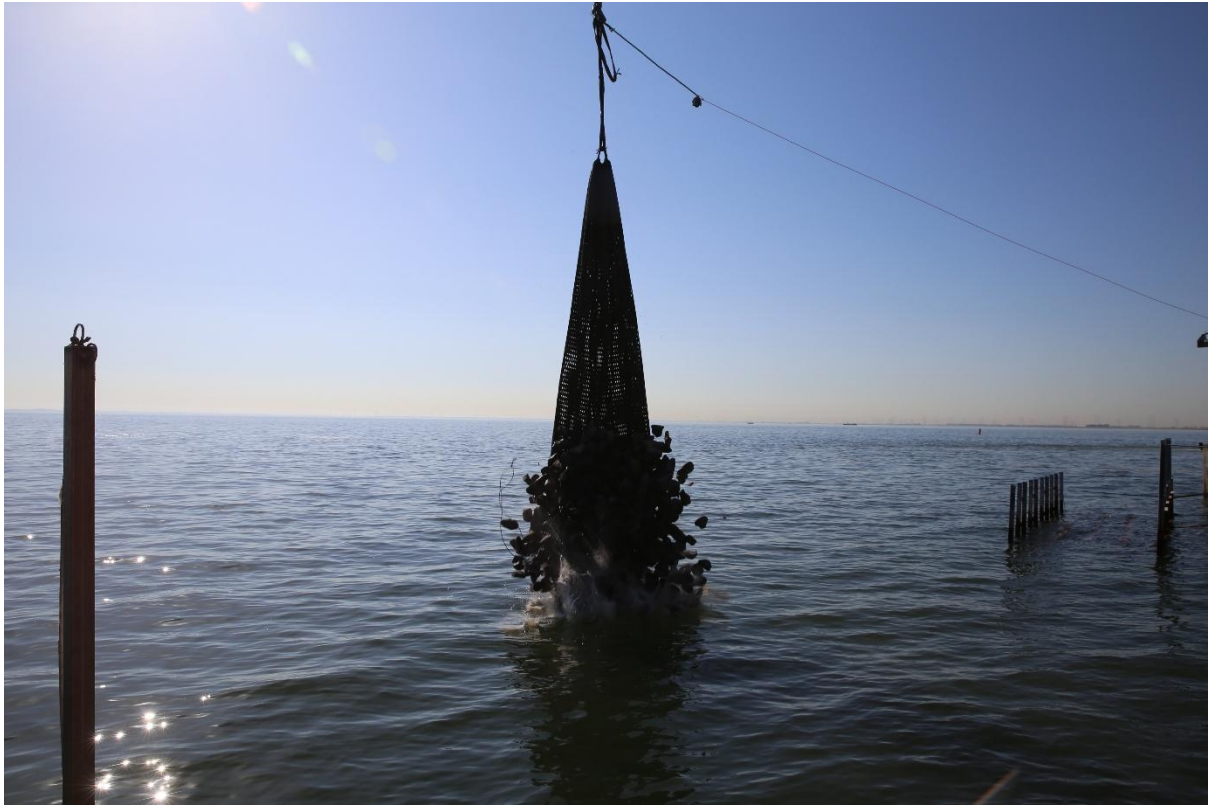
Figure 2-11. The moment of release of the rocks from the rock bag. Photo courtesy Gees van Hemert.
