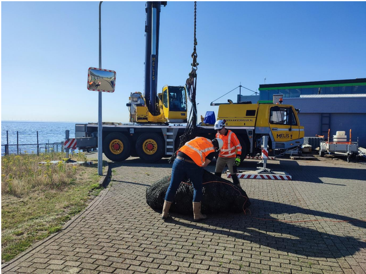
Figure 2-10. Crane in position with rock bag attached and being prepared for dropping.
