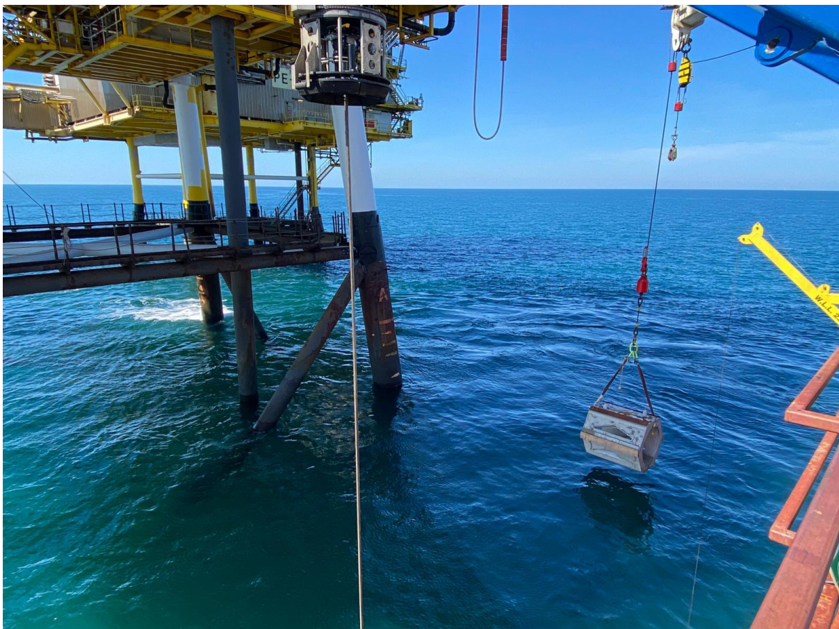
Figure 6. Deployment of one of 5 ExoLodge units beside the North Sea gas platform K5PK on 28 th July 2024.
